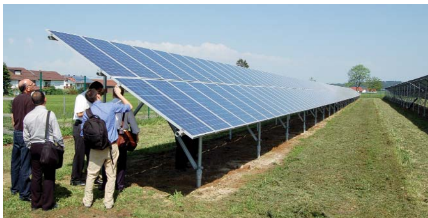
PV free-field installation of HAWI Energietechnik
